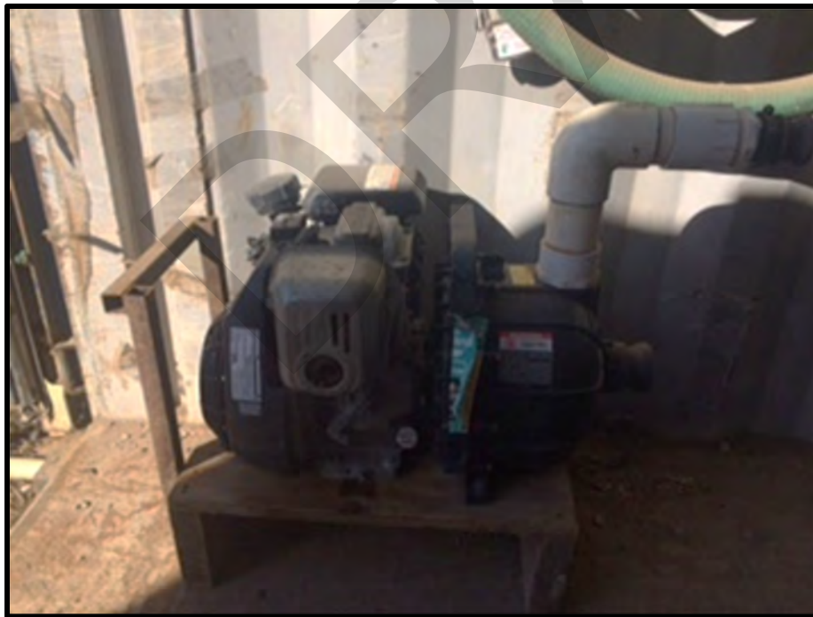
Figure 23. Pump used to Operate the Clam Rake
